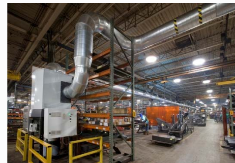
General Extraction & Circulation
