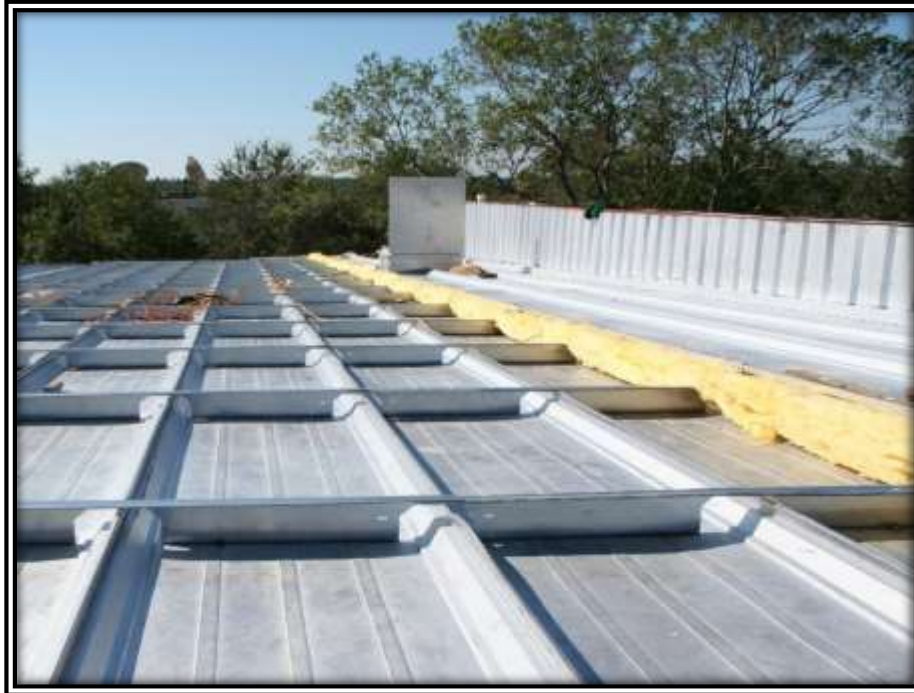
Photo L: Here a tall clip is being use in association with the notched purlin so that insulation can be incorporated into the new roof system.
