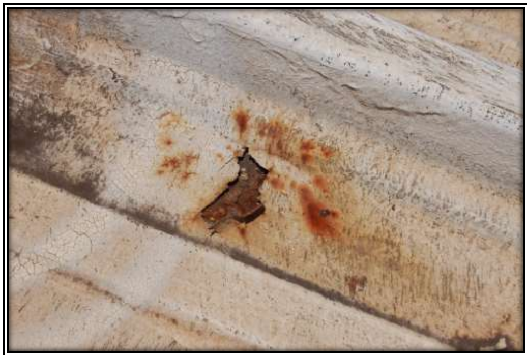
Photo F: Coatings that de-bond from the metal below can crack, allowing water to enter in below the coating and deteriorate the metal panel below.
