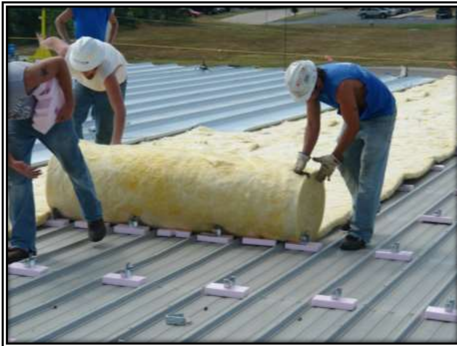
Photo M: Tall clips are being used to raise the height of the roof panel so that a layer of insulation can be installed.
