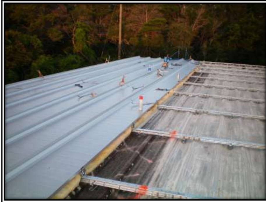
Photo N: New sub-purlins and insulation have been installed, which is then followed by the placement of the new roof panels.
