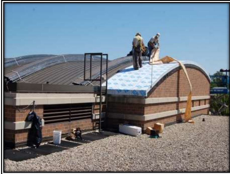
Photo I: The existing metal roof panels have been removed and underlayment installed. The bundled new metal roof panels have already been lifted to the roof and are ready for installation.
