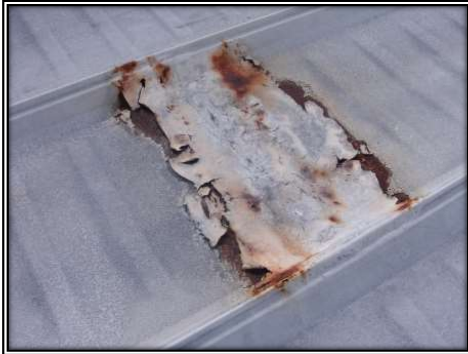
Photo H: Coating applied to the transverse lap seam, peeled and allowed moisture to enter under the coating, but not out. This resulted in the deterioration of metal roof panel.
