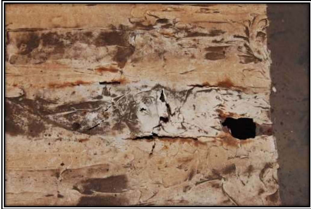
Photo G: The coating in this photo concealed a nearly rusted out panel that created a life-safety concern. The panel should have been repaired prior to coating.
