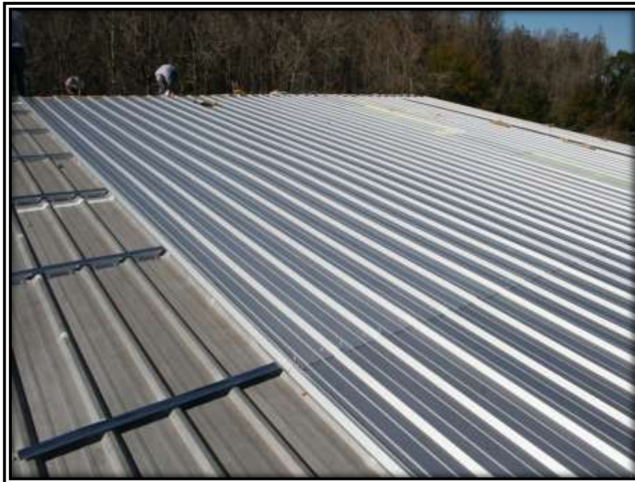
Photo K: Notched purlins placed over the existing standing seams in line with the purlins below is an efficient method to install a new roof panel.
