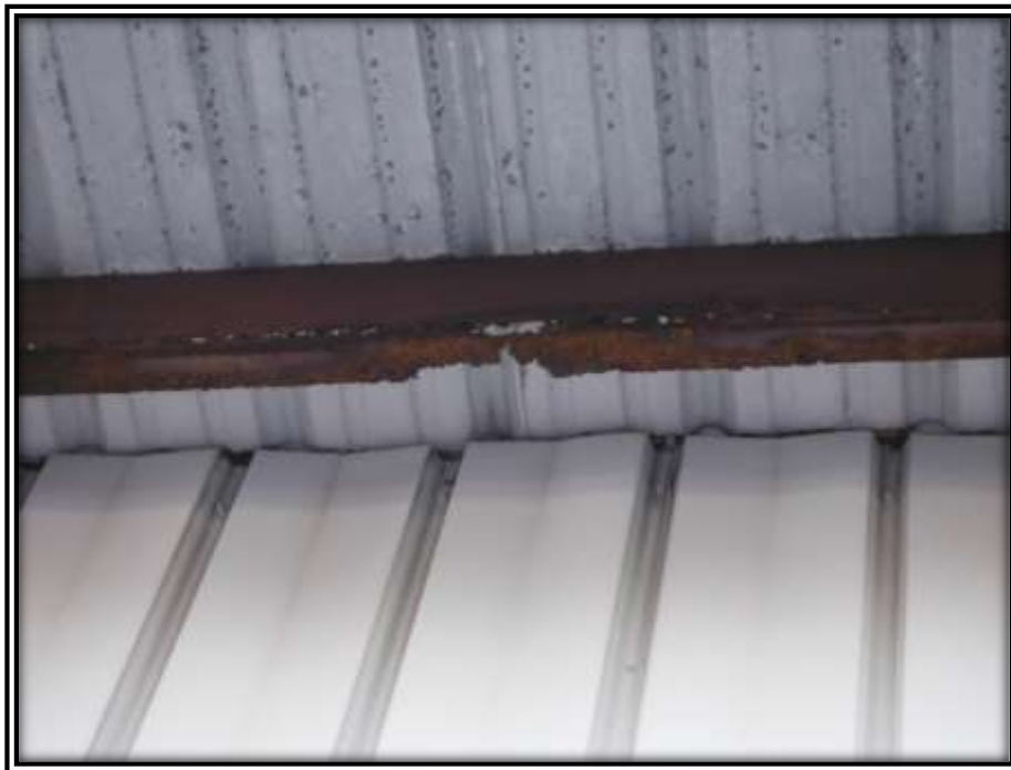
Photo E: Long-term moisture intrusion can have hidden life safety concerns as see in the photo above where the steel purlin has no structural integrity.
