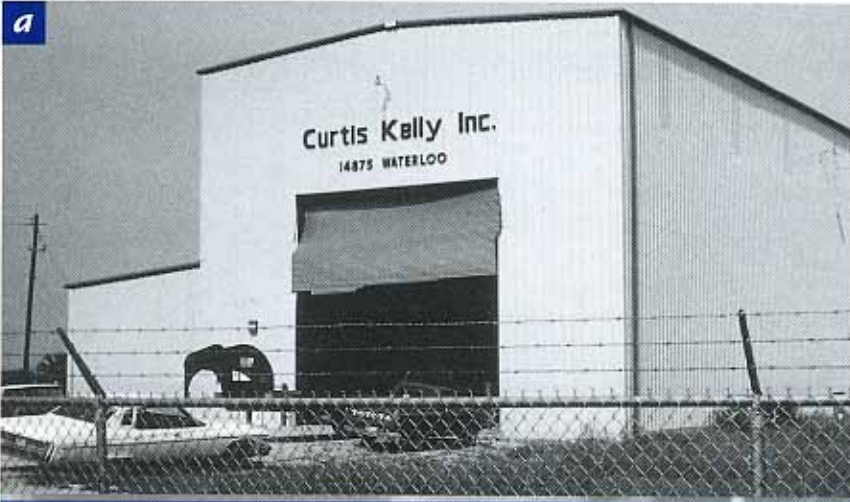
Photo 6: Observed damage to overhead doors a) Hurricane Alicia b) Hurricane Elena c) Hurricane Opal
