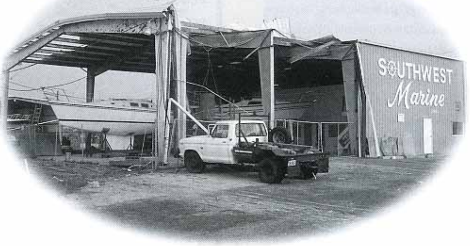
Photo 4: Hurricane Alicia Observation – Roof and wall damage to building with some open bays.
